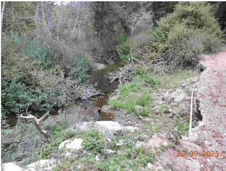
Photo 12. Mile 1.2, looking upstream from the edge of the eroded, reinforced road. Boulders to protect the road produce pool scour.
